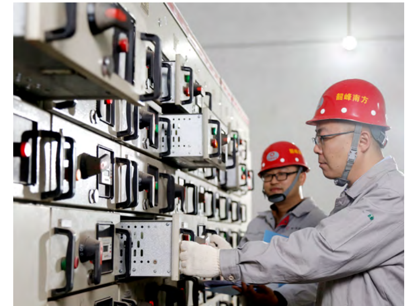
© Hunan Shaofeng South Cement Company Limited employees are checking the equipment in the electrical room
